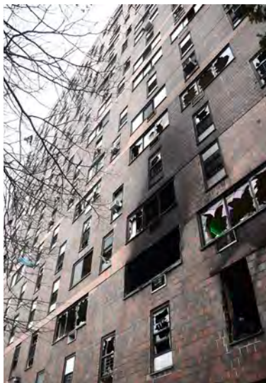
Exposure 3 side of the fire building.
