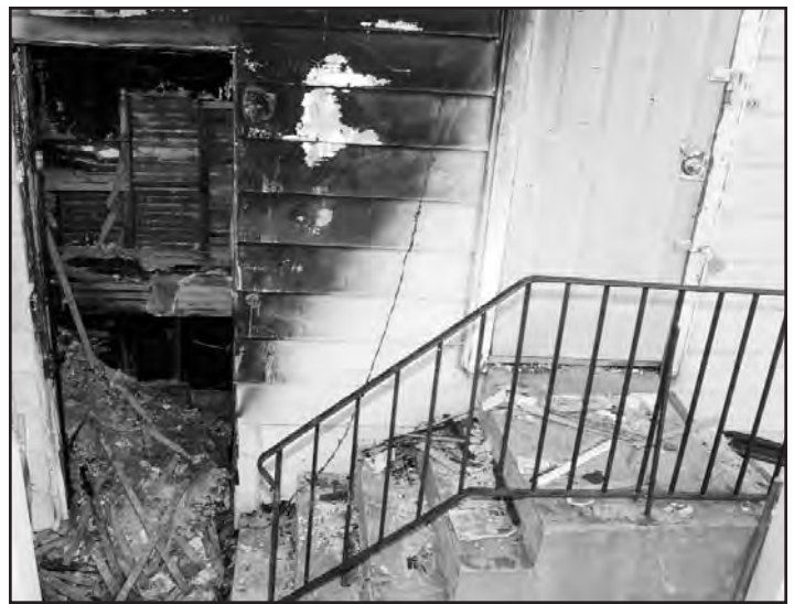
Photo #3--127-23 Hawtree Creek Road. The stoop and side cellar entrance on the same side of the building indicate an exterior entrance to the upper floor.
