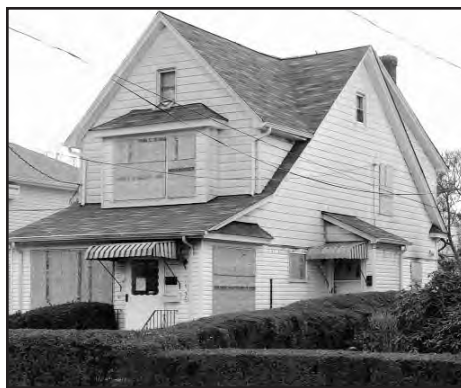
Photo #1--115-30 175th Street. The exposure #4 side entrance to the upper floors. There are very few windows on this side of the building, indicating stairs to the second floor run on the exposure #4 wall.
