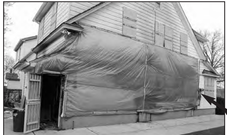
Photo #2--115-30 175th Street. Note the side cellar entrance with a few steps up to the kitchen and half flight down to the cellar. Also note the side cellar windows at ground level. The multiple meters (arrow) indicate multiple apartments.
