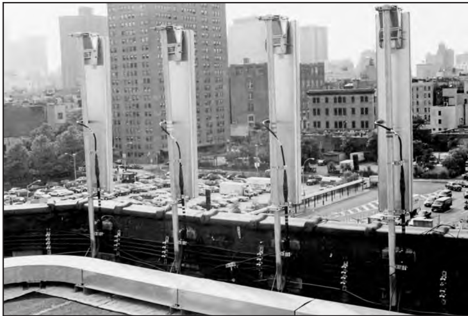
Unprotected coaxial foam radio frequency cable, originating from an interior base station, is fastened to the roof-side surface of the parapet wall where it connects to an antenna. Cable trays or raceways, also pictured, protect the coaxial cable, which travels across the roof surface.
