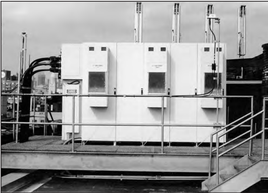
Roof-mounted base station (approximate weight is 20,000 lbs.) supported by two steel I-beams, which extend the entire width of the roof. The steel I-beams are pitch-pocketed into the two bearing walls of the building. Sometimes, the I-beams, measuring 10 inches, are secured to the building parapet. Metal grill surface surrounding the base station allows telecommunication workers to access all sides of the base station. It will, however, decrease the area of the roof Firefighters will be able to ventilate.
